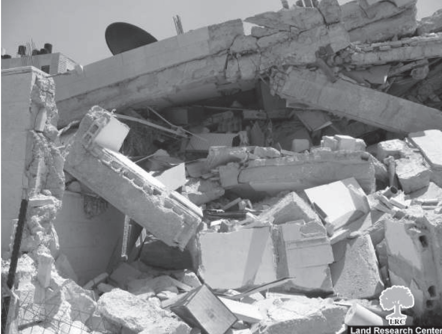
Abu Eishah building after being demolished by explosives, along with the furniture of the seven families living there
