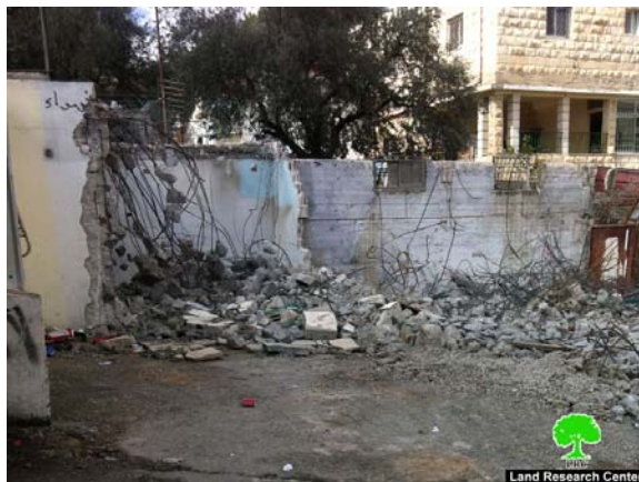
Demolished shop in Wadi Hilweh, Silwan. (February, 2012)
